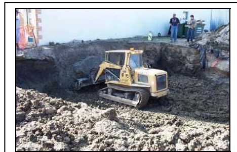
A leaking UST excavation. Source: http://www.epa.state.il.us/land/lust/ust-fund.html
