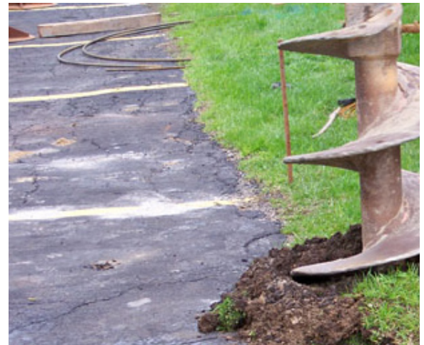
Ground-breaking commences after restaurant owner Brian Great secures permits from the Village of Schiller Park and the Federal Aviation Administration.
