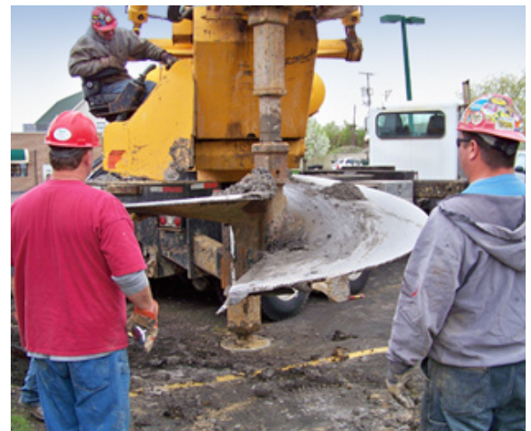
Two-thirds of the project's costs were for infrastructure, including a 30-foot foundation.
